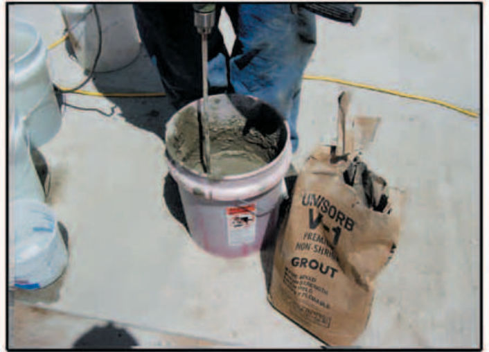
V-1 Grout mixed in a pail with a power drill and paddle.
