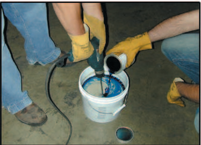
Standard V-100 Epoxy Grout mixed in a pail with a power drill and paddle.
